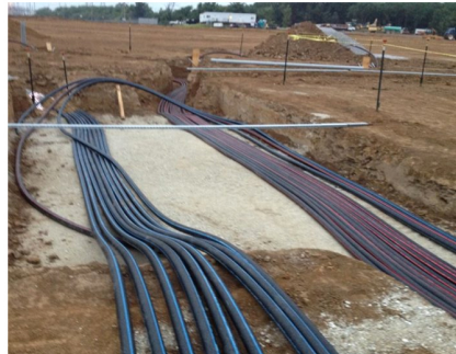
Communication pipeline on highway and rail way.
