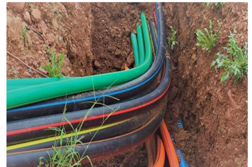
Other underground communication pipeline
