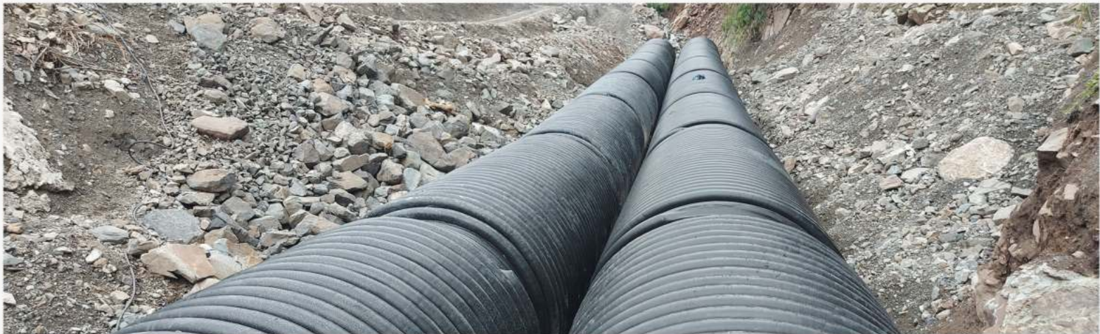
Penstock Pipeline for Hydropower
